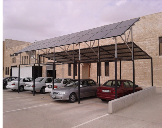
Figure 1. Solar PV parking installed at HU.
